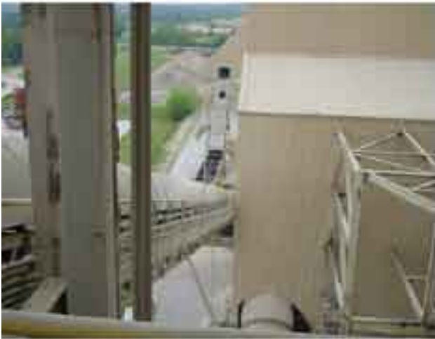
Conveyors to Kiln
