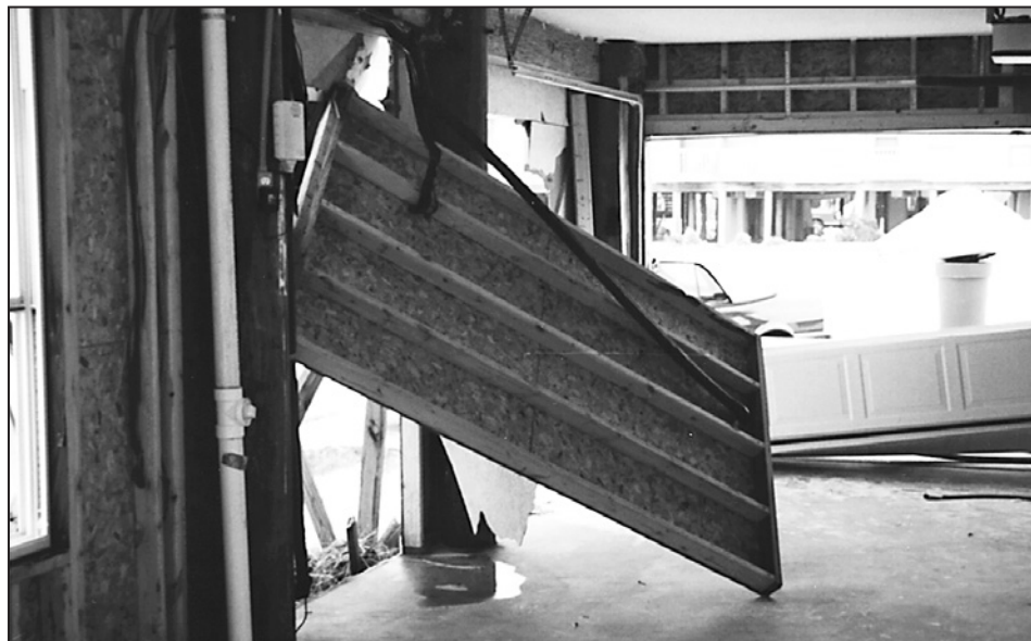
Figure 9-29. Breakaway wall panel prevented from breaking away cleanly by utility penetrations, Hurricane Opal (Florida, 1995)
