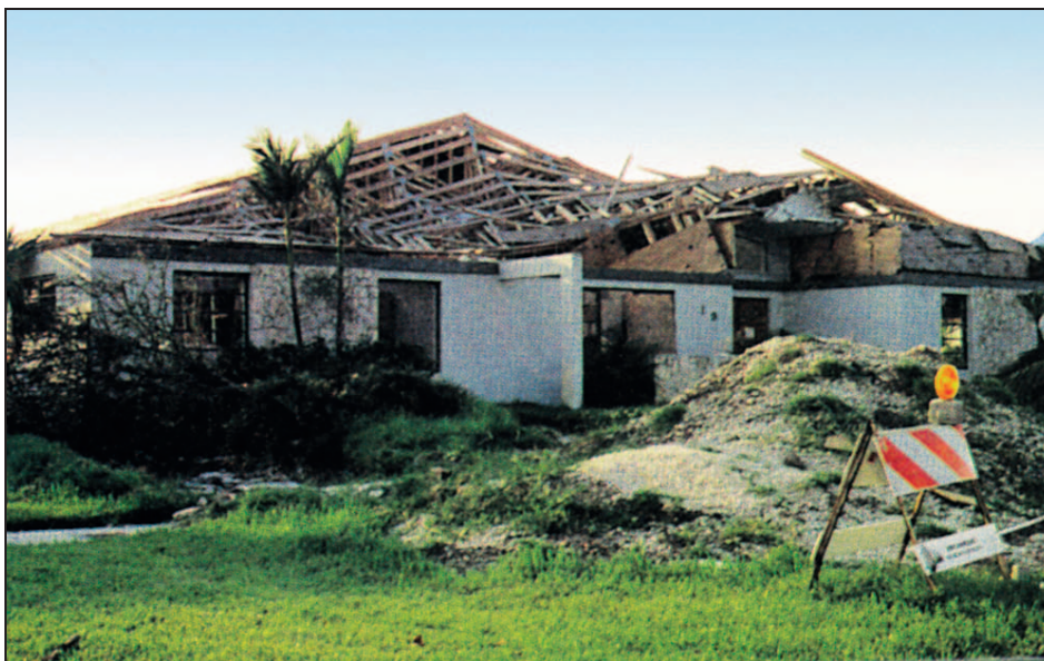
Figure 9-21. Gable-end failure, Hurricane Andrew (Dade County, FL, 1992)
