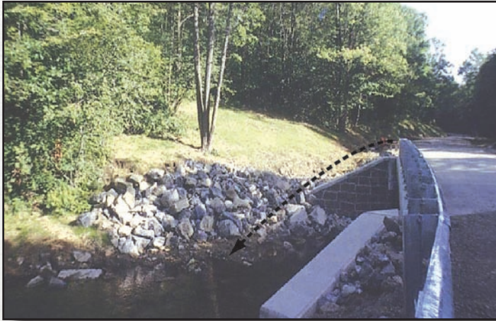
Figure 4.22a—Before: A typical crossing with ditches armored with rock and draining directly into the stream.
