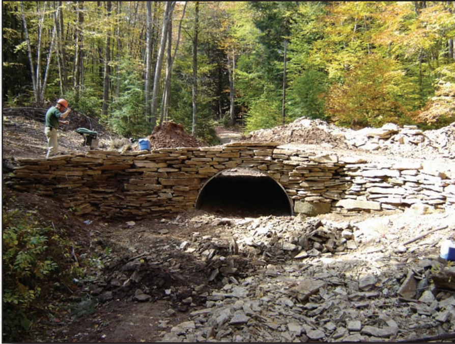
Figure 6.12—A bottomless arch pipe has just been installed over a currently dry stream channel.
