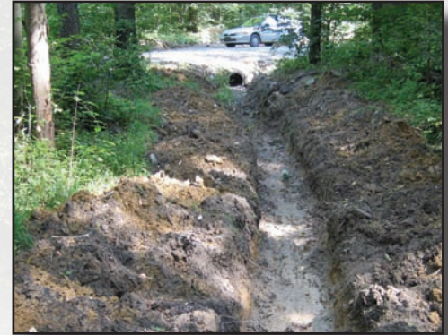
Figure 5.5—Traditional deep pipe. It has a long outlet trench requiring continual maintenance.
