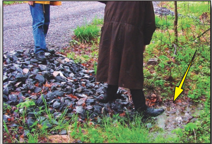
Figure 2.14—This is the same mattress outlet after completion. Notice the water flowing out of the mattress below the road.
