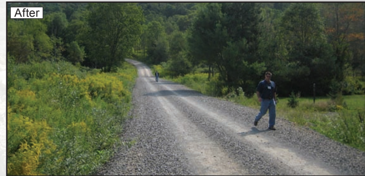
Figure 2.17 and 2.18—This roadway cuts across a flood plain wetland. A 300-foot-long French mattress was used to provide relief for wetland flows while providing a stable road base and preventing beavers from damming the nearby stream pipe.
