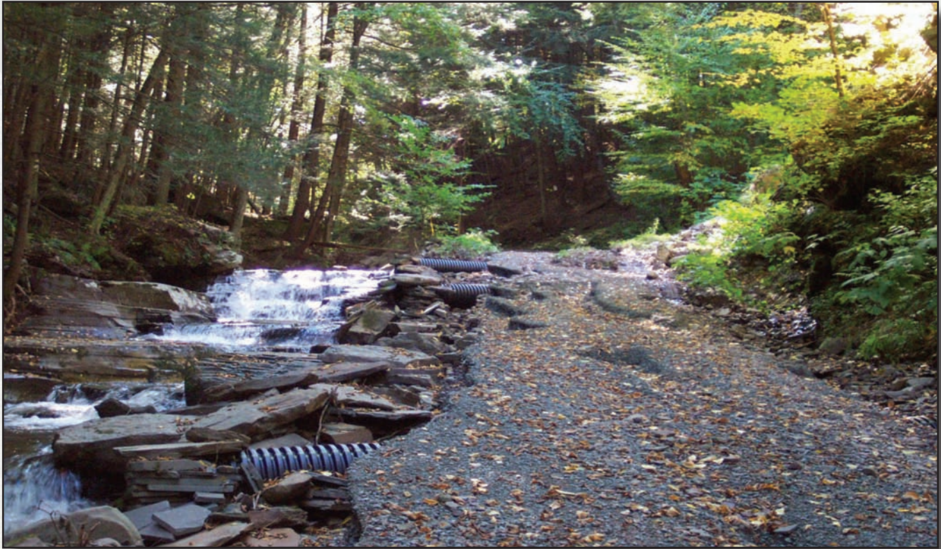
Figure 6.1—Consequence of poor road location results in loss of road and increases sediment delivery.
