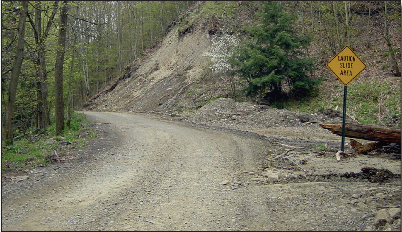
Figure 7.1—Unvegetated cutslopes are a source of sediment.
