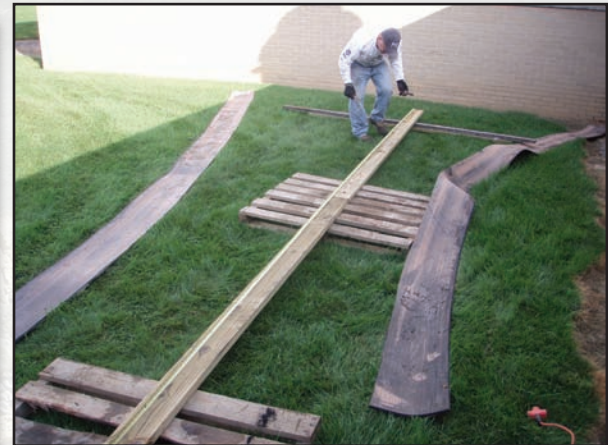
Figure 3.17—Construction of a 24-foot-length diversion. Note that the belt has been cut in half lengthwise. A 4-foot board on top of the belt spans the lumber joint of two 12-foot boards.
