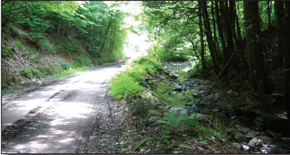
Figure 6.14—This road is constantly being eroded and flooded. Relocating the road away from the stream, while initially costly, will pay for itself in a few years of reduced flooding and repair costs.
