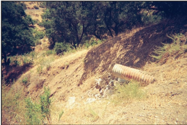
Figure 5.2—Shotgun culverts causes accelerated erosion.
