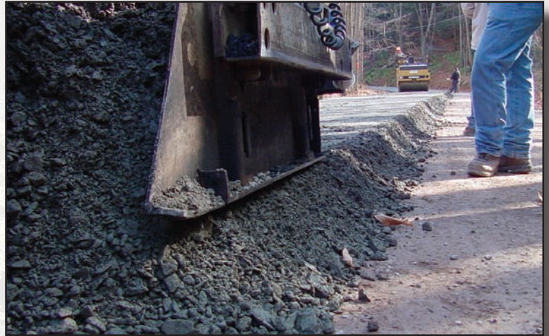
Figure 8.5—A well-graded aggregate is being placed through a paver at a noncompacted depth of 8 inches, and compacted to 6 inches. Notice the roller in the background for compaction.
