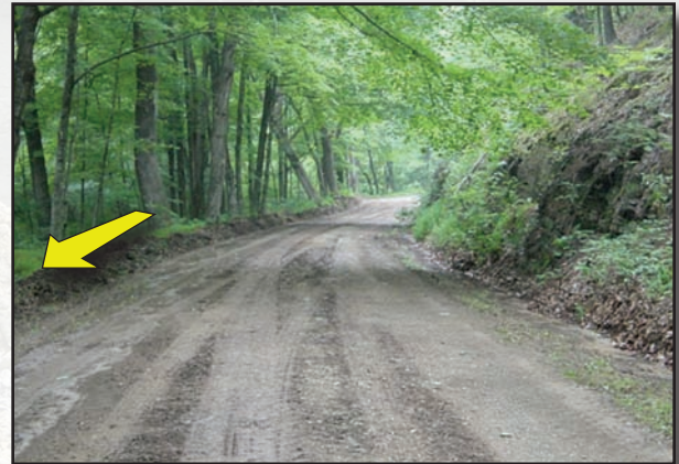
Figure 4.15—The berm was created by recent grading. Removing the berm and crowning the road allows sheet flow into the vegetation to the left.
