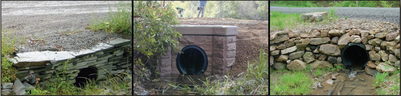
Figure 5.11—Headwalls come in various shapes, sizes, and materials, based on the situation and material available.
