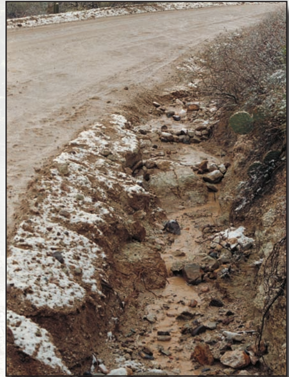
Figure 4.6—Eroded ditches are a common problem.
