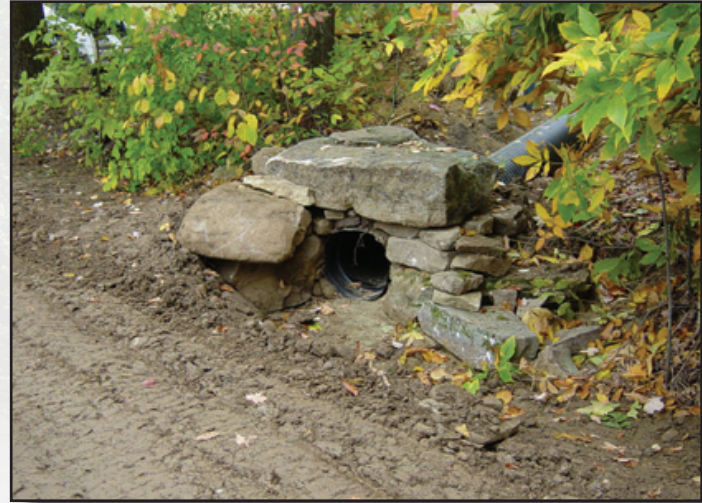
Figure 5.10—The inlet of a through-the-bank pipe shown during installation before the pipe is covered.
