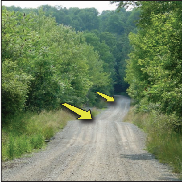
Figure 3.7—The two grade breaks pictured here prevent water from flowing down the road, even if the road's crown were to be lost.
