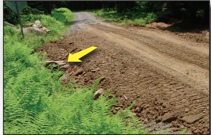
Figure 5.8—The same pipe is shown here covered with fill, before final compaction. Arrow denotes headwall or pipe inlet.
