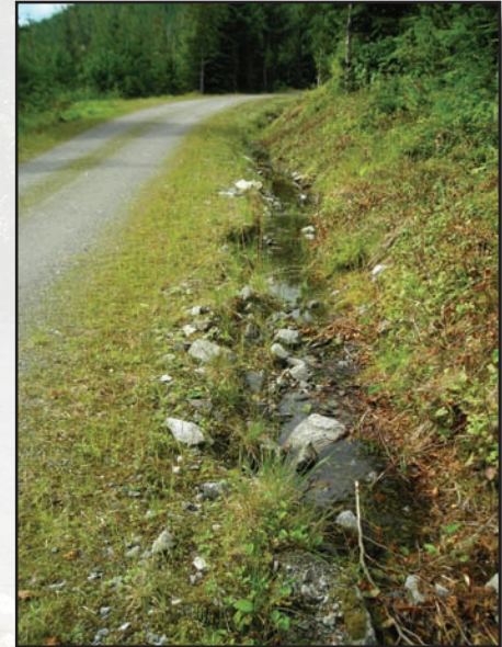
Figure 2.4—Road ditch with standing water.
