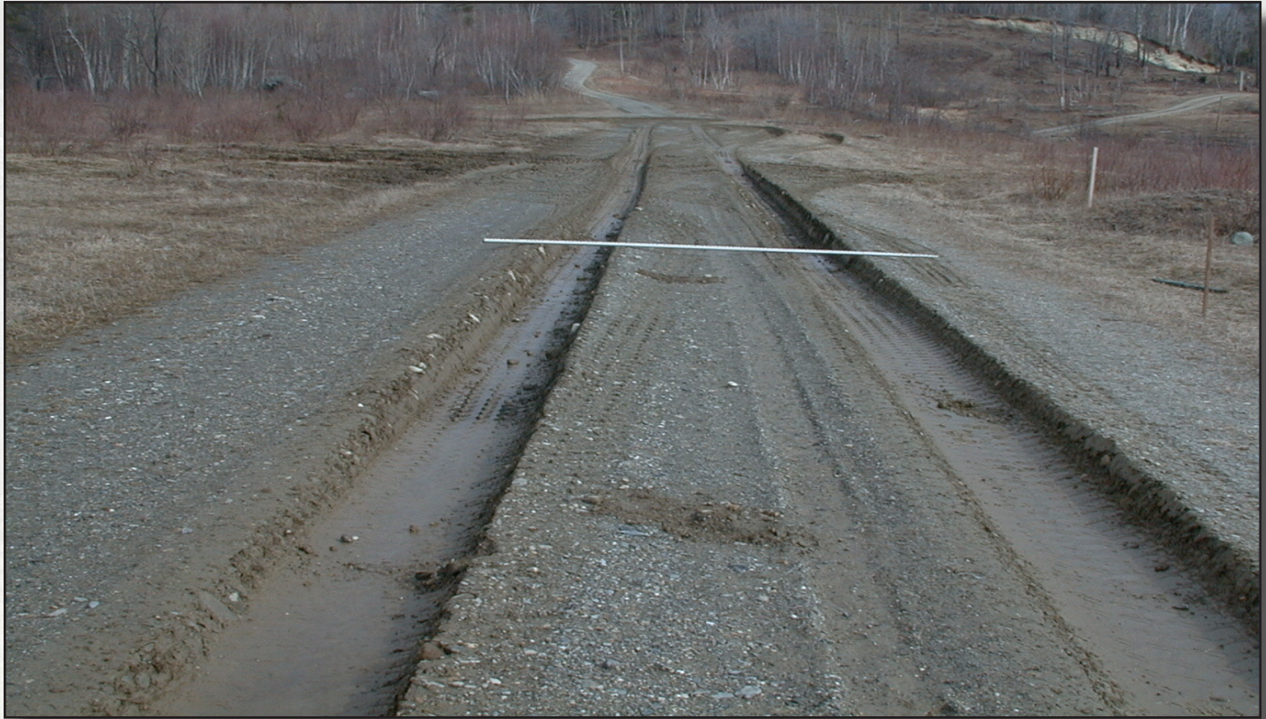
Figure 8.1—Proper gradation of aggregate can prevent the raveling and pumping in this picture.
