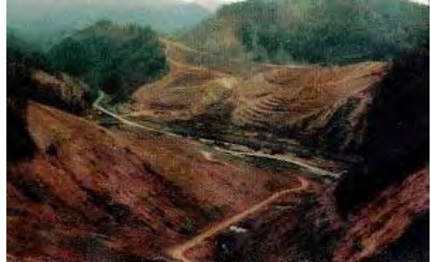
Terraces can be incorporated into the grading plan to shorten the length of the slope and to reduce the velocity of storm water flows (Source: Boaze et. al, 2000)
