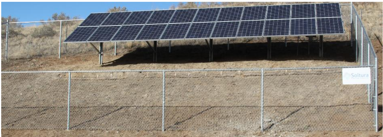
Figure 6. PV Array with Fence
