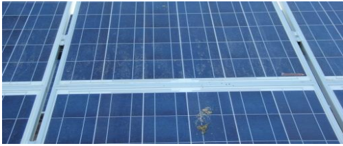
Figure 3. Presence of bird's waste on PV module
