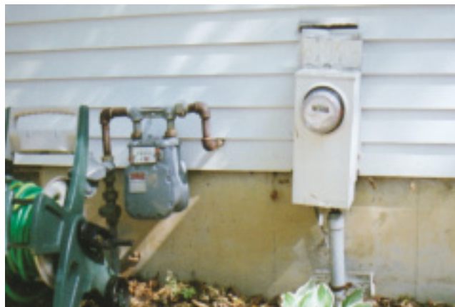
Figure 5.4: An electrical service box torn from a home because of soil settling.
