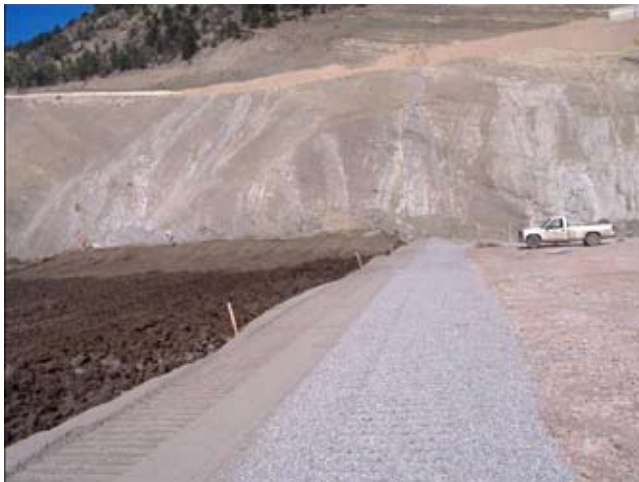
(g) Earthfill is compacted on both sides of the filter zones that have been laid. The process is then repeated as the embankment is raised.
