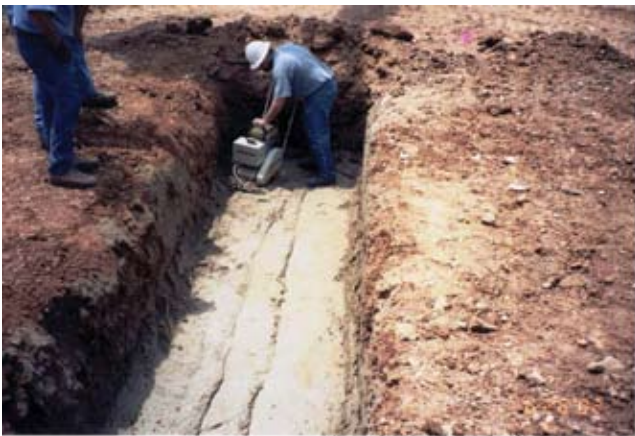
(c) Step 1 in constructing filter diaphragm. Trench has been excavated below grade at location of principal spillway conduit, and sand filter is being compacted in the trench. Conduit will be laid on top of trench after it is filled with filter material compacted to the required degree excavated and backfilled with sand.
