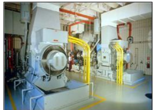
Gas turbine engine designed to use LFG
