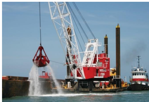
The image above shows a dredging operation consisting of a clamshell bucket dredge on a barge
