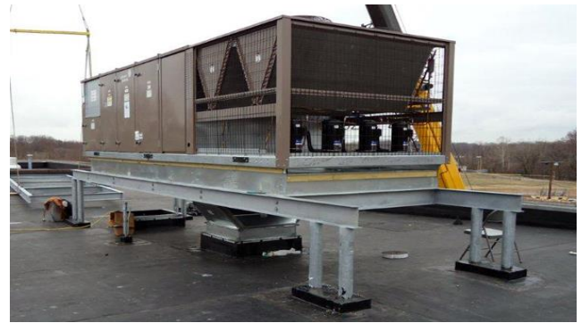
Rooftop mounted AC Chiller System
