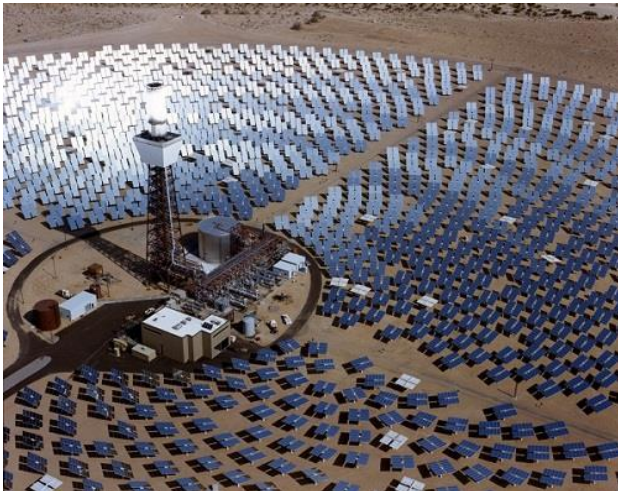
Receiver Tower with a surrounding field of Heliostat Structures
