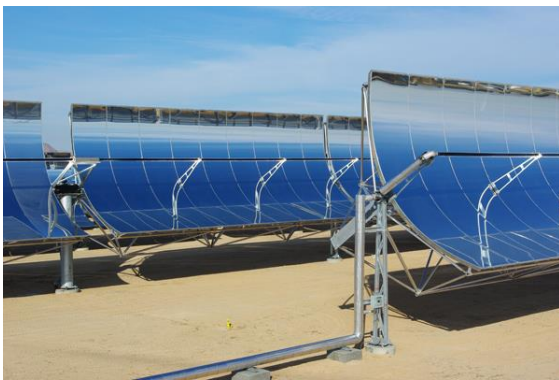
Parabolic Trough Mirrors Image Source: Skyfuel.com
