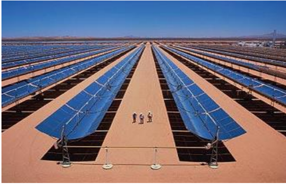
Parabolic Trough Collectors at SEGS III to VII – Kramer Junction, CA
