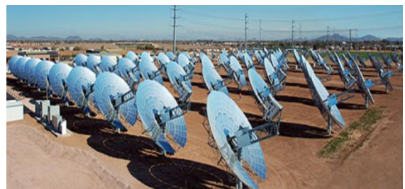
Maricopa Solar SunCatcher units Image source: Tessera Solar
