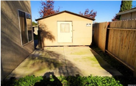
Shed and Concrete Pad built right up to fence Image Source: Movato.com
