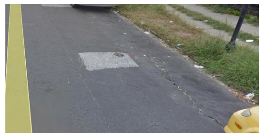
Linear Cracks in the Pavement (observed prior to collapse) Image source: Google Earth
