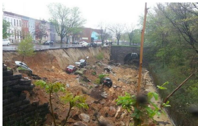
Aftermath of the Retaining Wall Failure
