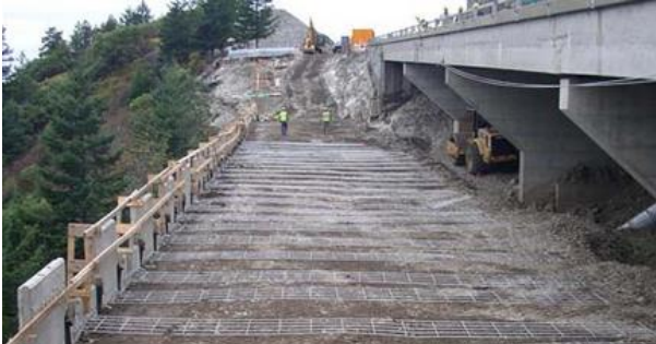
Mechanically Stabilized Earth Wall (using steel mesh) (Note how the bar mat is affixed to the concrete facade panels)
