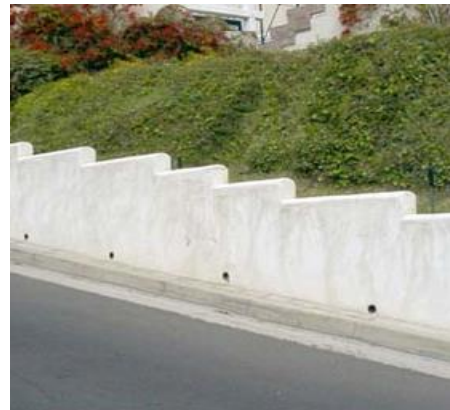
Example of Weepholes - 3" Diameter
