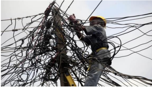
Nigerian Power Pole with Illegal Taps Image Source: voanews.com
