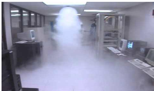
Total CO2 Flooding of a Server Room Image Source: cubefireandsecurity.com
