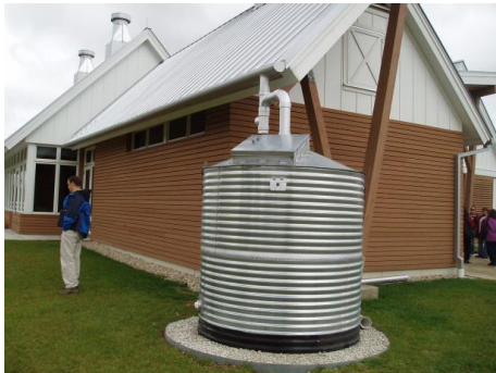
Ground Level Rainfall Cistern
