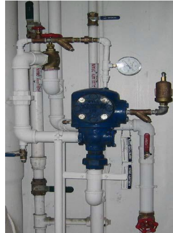
Dry Pipe System Exhauster (the blue component)
