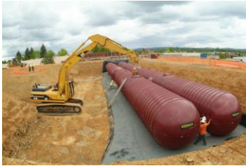
Underground Storage Tanks Image Source: xerxes.com
