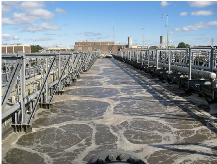
Activated Sludge Aeration Tank
