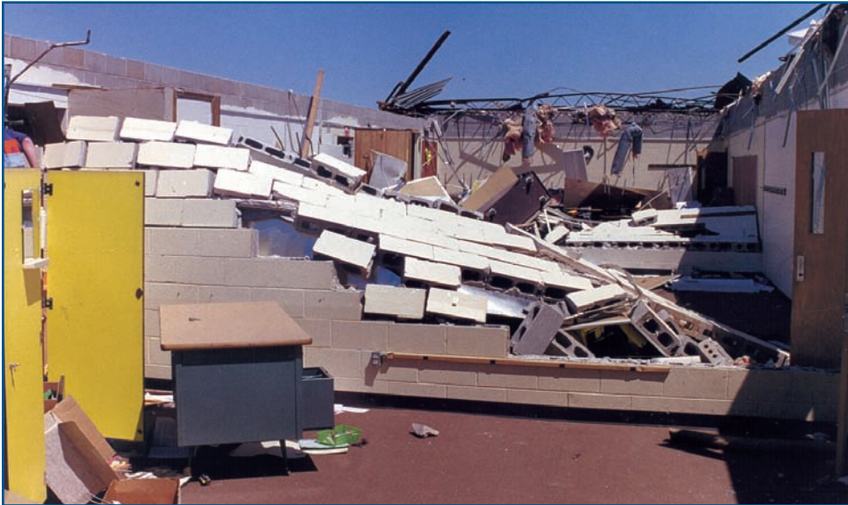
Figure 3-17 Interior and exterior unreinforced masonry walls were damaged when reinforced bond beams failed.
