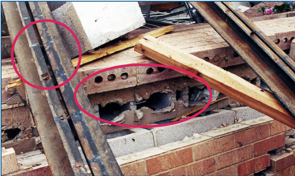
Figure 3-21 Failed roof structure showing broken welds between metal roof deck and tops of joists (upper circle) and lack of vertical reinforcement (bottom circle).
