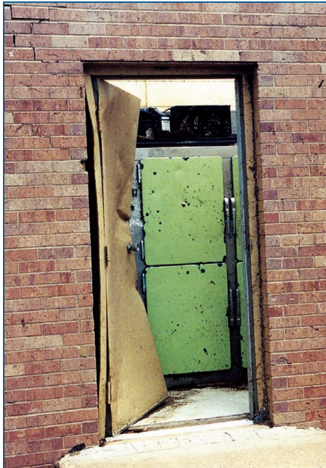
Figure 2-3 Example of severe damage from a windborne missile. This metal door was pushed inward by the impact of a heavy object.
