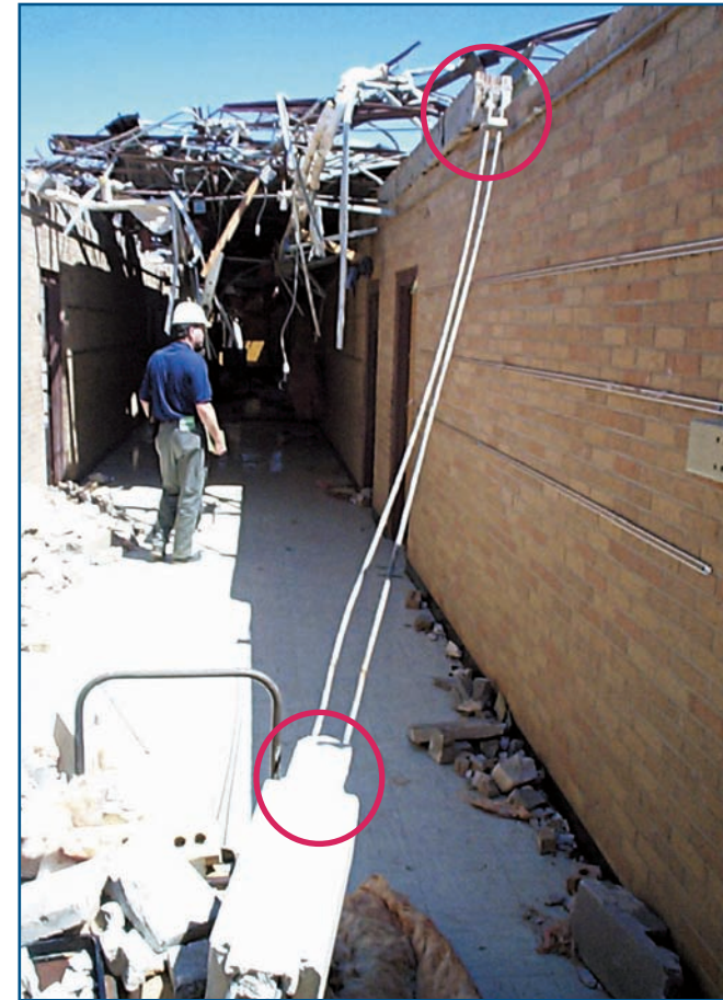
Figure 3-18 Corridor area. Separation of reinforced bond beam (indicated by circles) from supporting wall.
