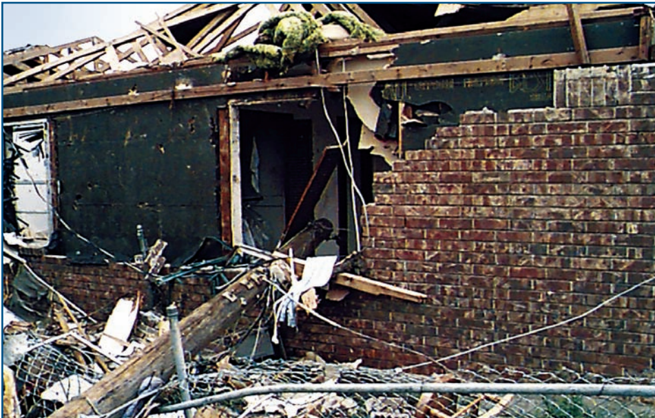
Figure 4-4 This power pole penetrated a window and extended several feet into the house after being blown 40 feet from its original location.
