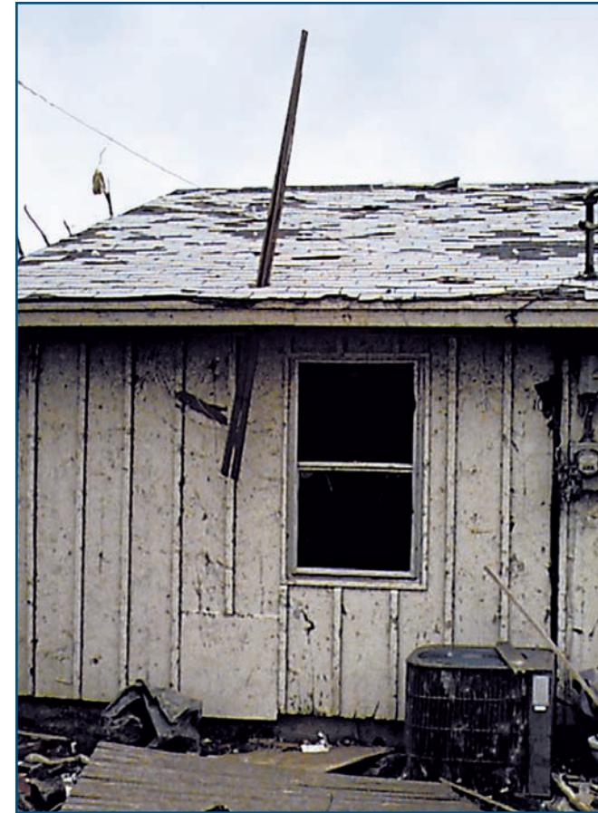
Figure 4-5 This photograph illustrates the importance of overhead protection in refuge areas. The missile shown here fell nearly straight down.
