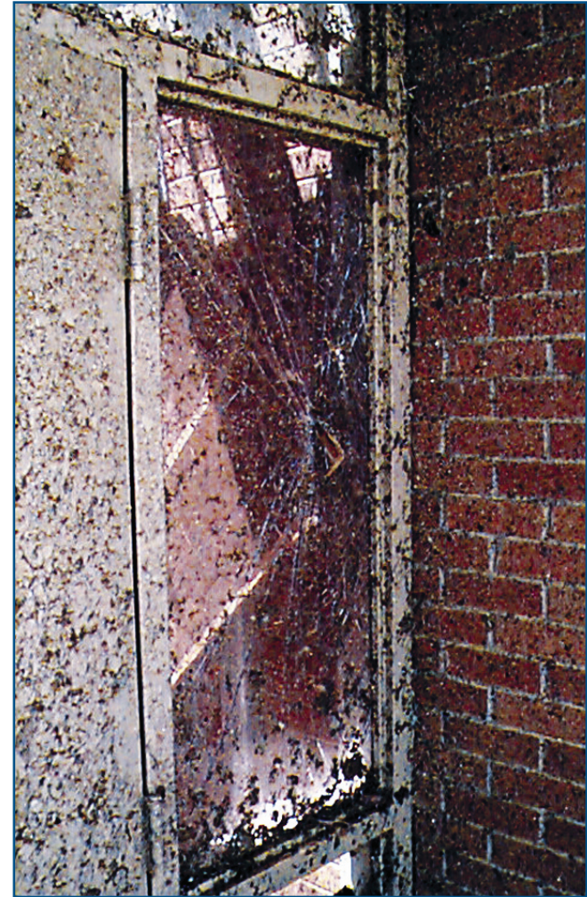
Figure 3-22 Impact performance of laminated glass. The corner of a table penetrated this laminated glass window, but the glass remained in its frame.
