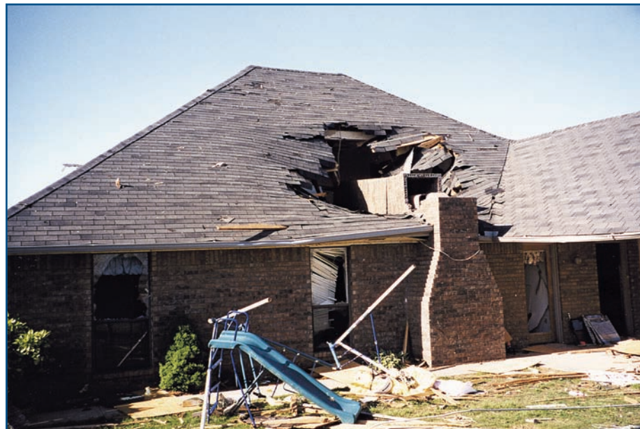
Figure 4-3 Failure of brick chimney under tornado winds damaged the room of this house in Moore, Oklahoma.
