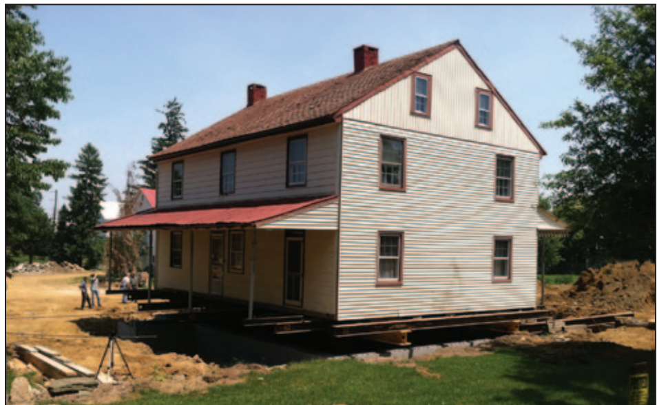
Figure 5R-13. House is lowered and connected to the foundation after foundation walls are completed (photo courtesy of Wolfe House Movers)
