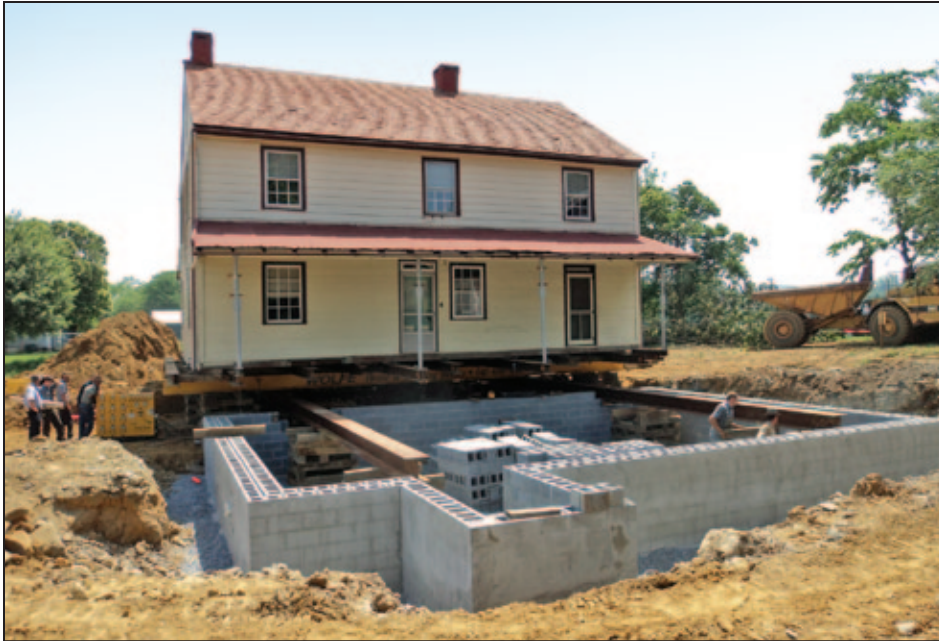
Figure 5R-10. New foundation wall construction begins (photo courtesy of Wolfe House Movers)
