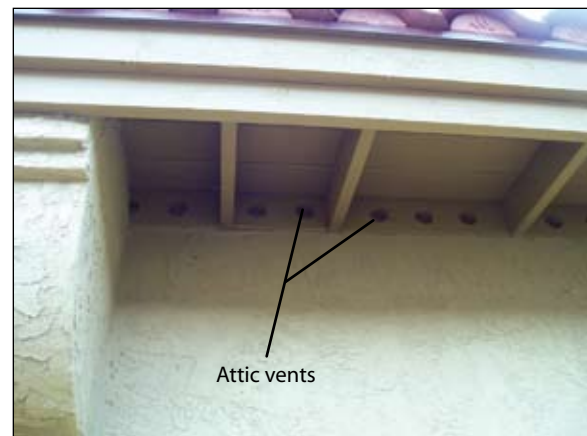
Figure 1. An open overhang. The exposed timber rafters and decking are susceptible to ignition, and embers and hot gases can enter the attic through unprotected vents.
