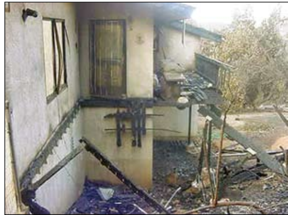
Figure 5. Combustible debris under this deck ignited and led to the destruction of the deck. Although the siding is noncombustible, the fire spread from the deck through a window to the interior (firecenter.berkeley.edu).
