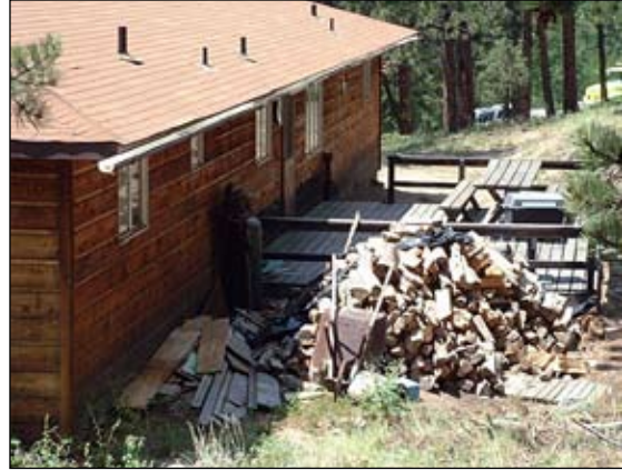
Figure 2. Combustible materials adjacent to a building create a hazard (Anchor Point Group, Boulder, CO).
