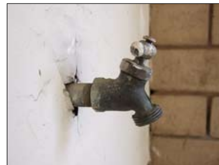
Figure 1. The gap around utility penetrations such as this one should be filled.
