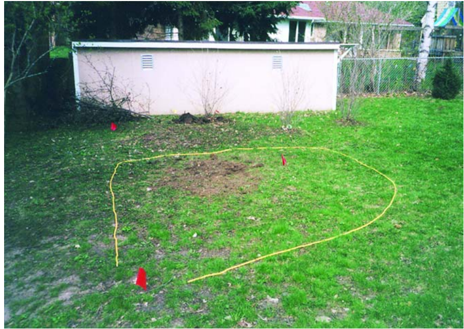
The perimeter of a rain garden is defined with string before digging.
