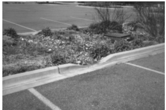
Figure 4. Bio-retention median or rain garden in Maryland with overflow drain visible on the right. The top of the overflow, shown here as a metal grate, is typically 9 inches above the bottom elevation of the bio-retention area.
