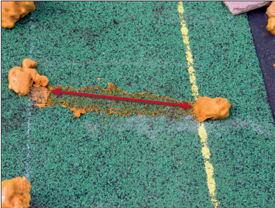
Figure 11-44. Adhesive that debonded from the cap sheet
