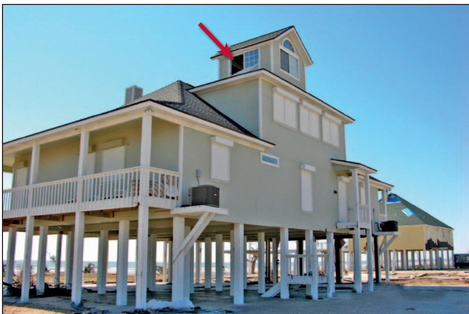
Figure 11-10. Unprotected cupola window that was broken. Estimated wind speed: 110 mph. Hurricane Ike (Texas, 2008)
