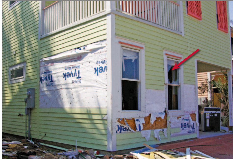
Figure 11-16. Blown-off fiber cement siding; broken window (arrow). Estimated wind speed: 125 mph. Hurricane Katrina (Mississippi, 2006)
