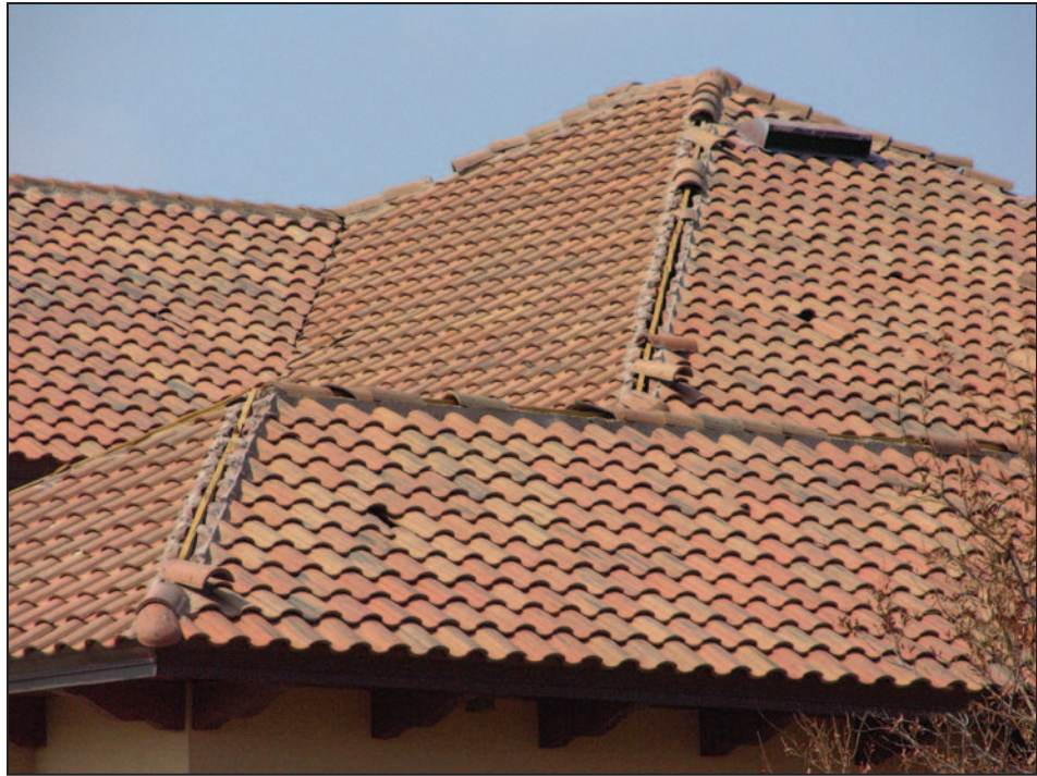
Figure 11-46. Blow-off of hip tiles that were nailed to a ridge board and set in mortar. Hurricane Ivan (Florida, 2004)
