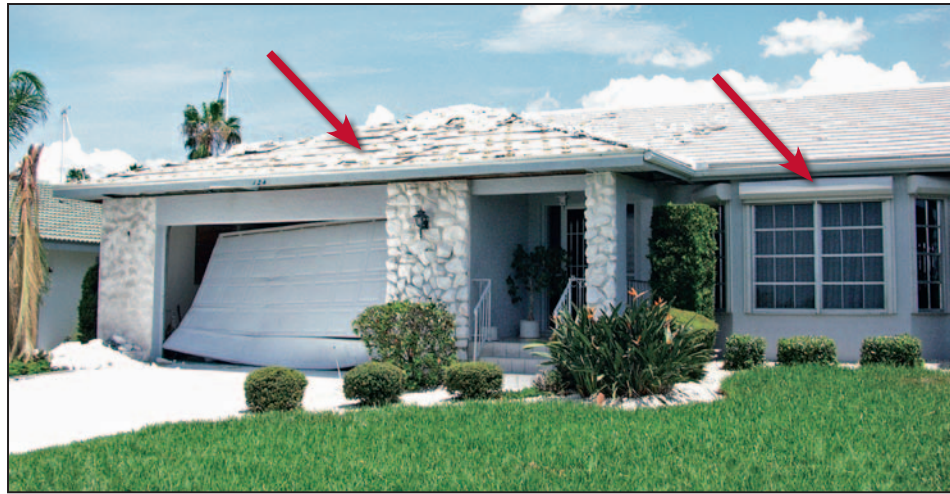
Figure 11-6. Garage door blown from its track as a result of positive pressure. Note the damage to the adhesive-set tiles (left arrow; see Section 11.5.4.1). This house was equipped with roll-up shutters (right arrow; see Section 11.3.1.2). Estimated wind speed: 140 to 160 mph. Hurricane Charley (Florida, 2004)
