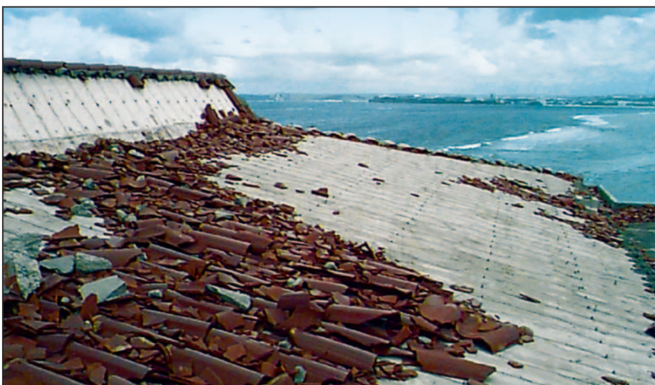
Figure 11-41. Blow-off of wire-tied tiles installed over a concrete deck. Typhoon Paka (Guam, 1997)
