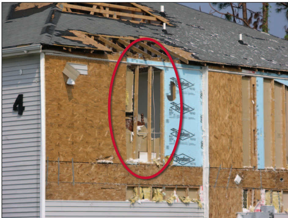
Figure 11-15. Blown-off vinyl siding and foam sheathing; some blow-off of interior gypsum board (circle). Estimated wind speed: 130 mph. Hurricane Katrina (Mississippi, 2006)
