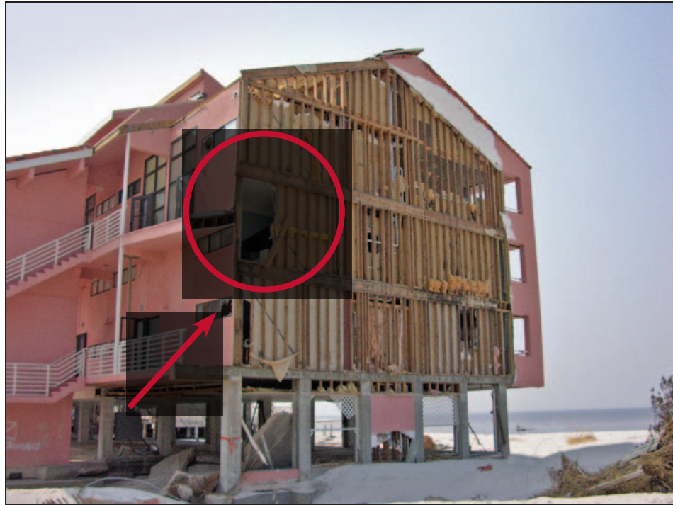
Figure 11-19. Blown-off EIFS, resulting in extensive interior water damage; detachment of the gypsum board or stud blow off (circle); two windows broken by debris (arrow). Estimated wind speed: 105 to 115 mph. Hurricane Ivan (Florida, 2004)
