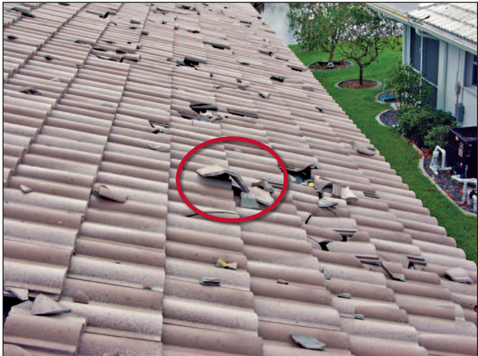
Figure 11-47. Damage to field tiles caused by tiles from another area of the roof, including a hip tile (circle). Estimated wind speed: 140 to 160 mph. Hurricane Charley (Florida, 2004)
