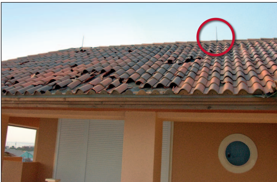
Figure 11-48. The fastener heads on this mechanically attached tile roof had corroded; air terminals (lightning rods) in a lightning protection system (circle). Hurricane Ivan (Alabama, 2004)
