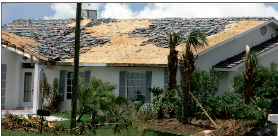
Figure 11-40. Large area of blown-off underlayment on a mortar-set tile roof. The atypical loss of waterproofing tile underlayment resulted in substantial water leakage into the house. Estimated wind speed: 140 to 160 mph. Hurricane Charley (Florida, 2004)
