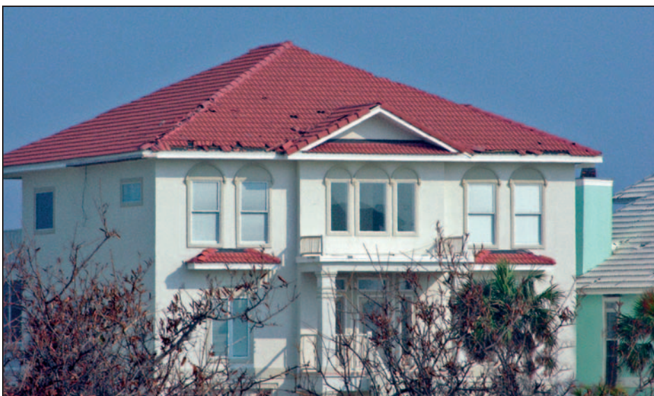
Figure 11-39. Blow-off of eave and hip tiles and some broken tiles in the field of the roof. Hurricane Ivan (Alabama, 2004)
