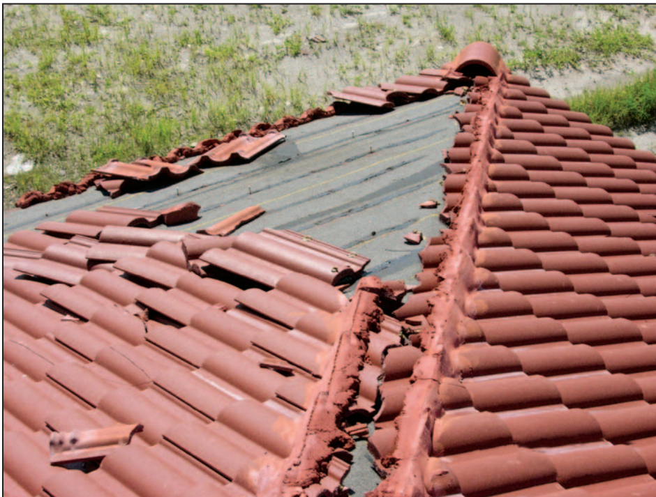
Figure 11-45. Blow-off of mechanically attached tiles. Estimated wind speed: 140 to 160 mph. Hurricane Charley (Florida, 2004)
