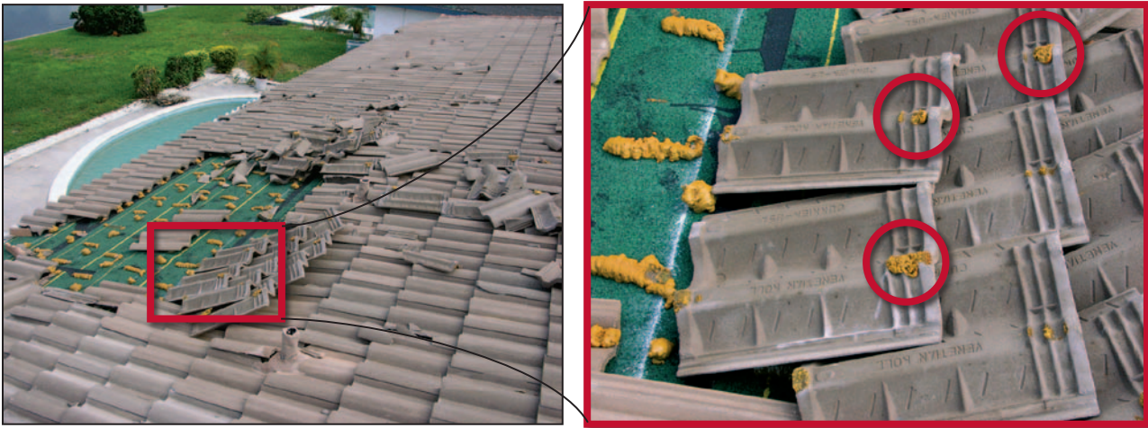
Figure 11-43. Blown-off adhesive-set tile. Note the very small contact area of the foam at the tile heads (left side of the tiles) and very small contact at the nose (circles). Estimated wind speed: 140 to 160 mph. Hurricane Charley (Florida, 2004)
