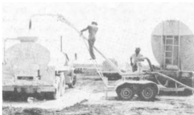
Figure 4-30. Jet slurry mixing plant.
