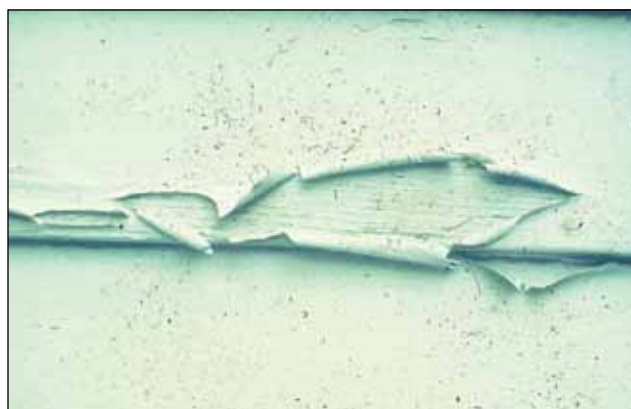
Figure 16-23. Intercoat peeling of paint, usually caused by poor preparation of old paint surface or excessive weathering of primer prior to application of top coat.
