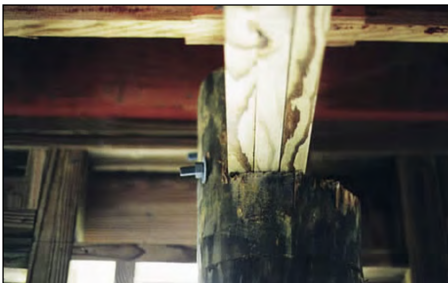
Figure 13-3 Overnotched pile. Also note mislocated bolt.
