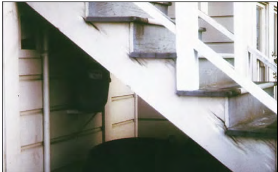
Figure 13-17 Deterioration in a notched stair stringer.
