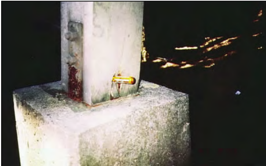
Figure 13-13 Wood decay at the base of a post supported by concrete.
