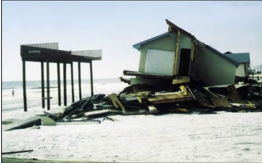
Figure 13-29 Building damage from Hurricane Opal at Pensacola Beach, Florida. The deck, which was constructed to State of Florida Coastal Construction Control Line (CCCL) design requirements, survived; the building, which was not constructed to CCCL requirements, did not survive. See Appendix G for a discussion of the Florida CCCL.
