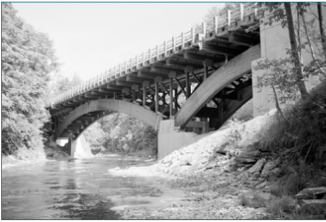
Figure 17–10. The Alton Saylor Memorial Bridge is a glulam deck arch bridge crossing Joncy Gorge in Angelica, New York. The center three-hinged arch spans 52 m (171 ft) and is the longest clear span in the United States. (Photo courtesy of Laminated Concepts, Inc., Big Flats, New York.)
