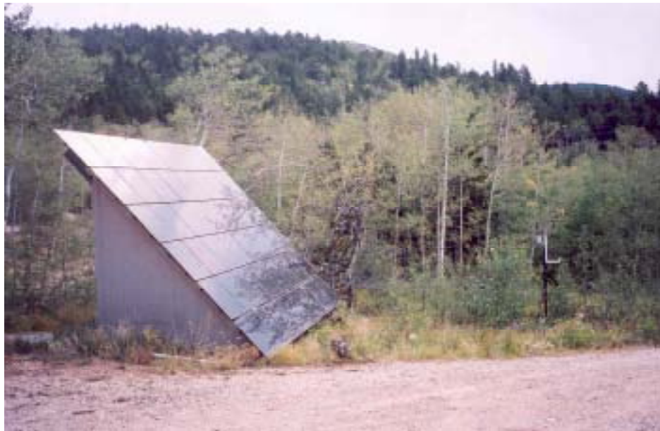
Figure 6.4. PV array (shown as roof of shed) and weather station (located on right of photo)
