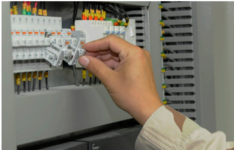
The Direct Digital Control (DDC) panel controls power for all heating, ventilation and air conditioning systems.
