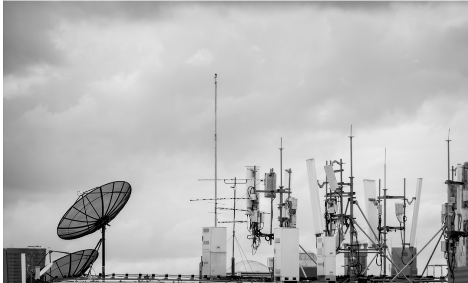
Telecommunication equipment for 5G radio network
