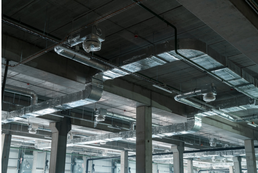
HVAC system layout on the ceiling of a warehouse
