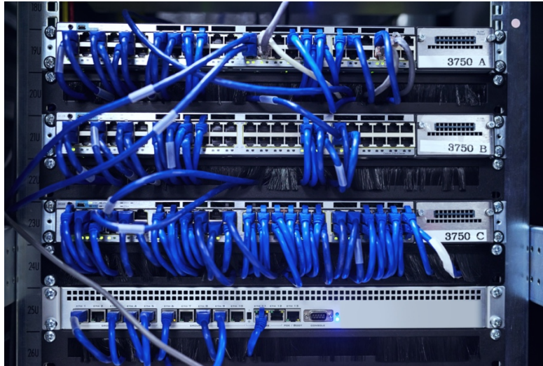
Network patch panel
