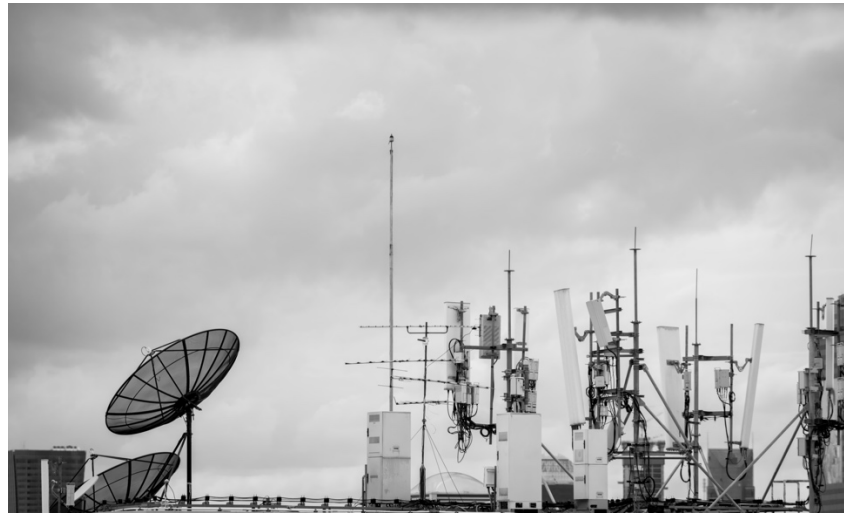
Telecommunication equipment for 5G radio network
