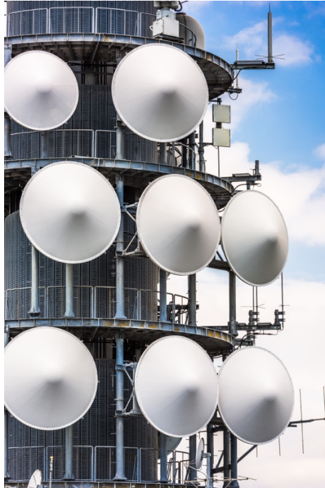
Telecommunications tower and infrastructure
