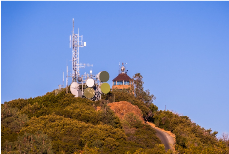
Telecommunication tower with parabolic antenna (dishes) for point-to-point microwave relay links.
