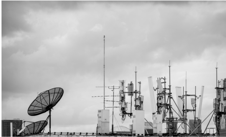
Telecommunication tower, antenna, and satellite dish for 5G radio network
