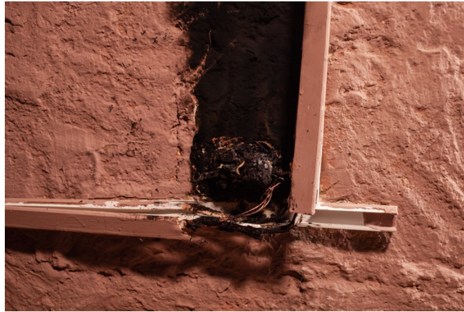
Burnt and melted electrical outlet
