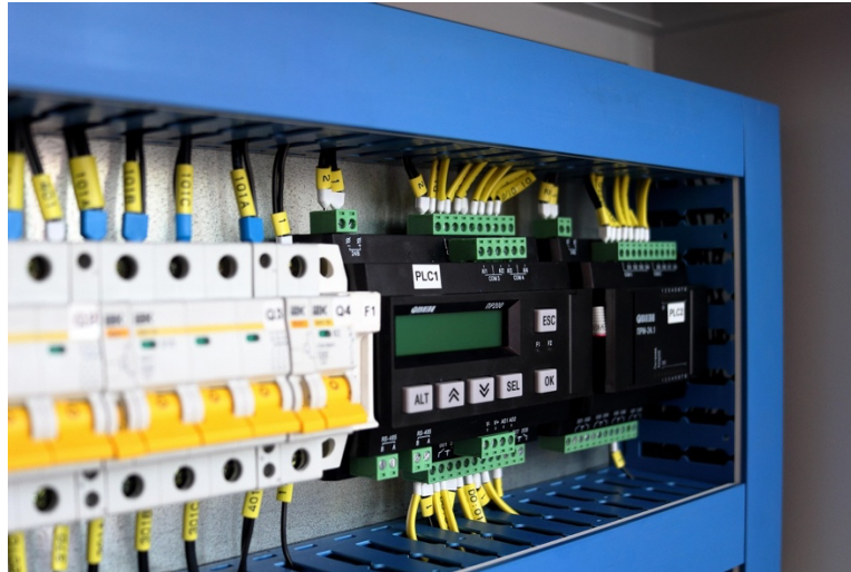
Programmable logical controller (PLC)
