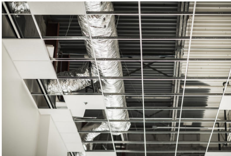
Air supply and conditioning duct of HVAC ceiling installation
