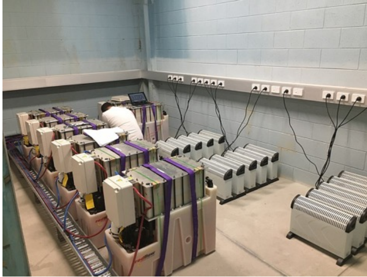
Zinc-bromine flow batteries, along with an energy discharge load bank (electric heaters)
