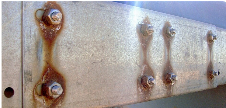
Galvanic corrosion due to differing anodic index between the bolts and the plate (D3j4vu at English Wikipedia, via Wikimedia Commons)
