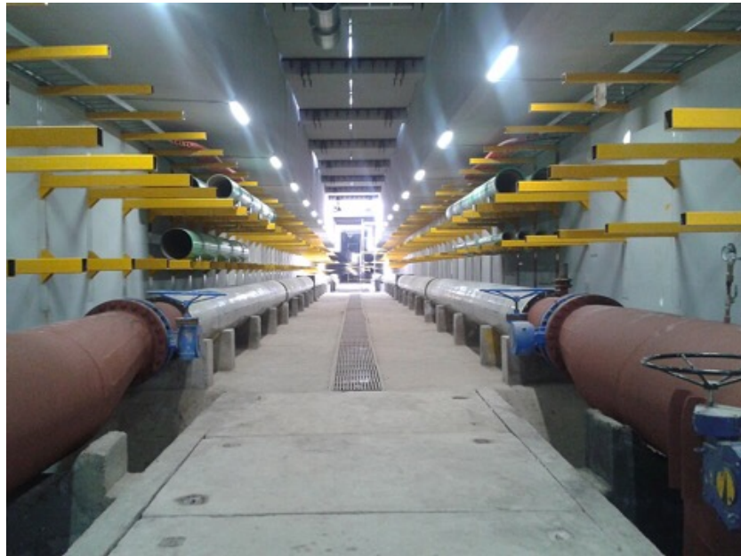
Figure 1: Underground utility corridor (Atul Tegar, CC BY-SA 4.0, via Wikimedia Commons)
