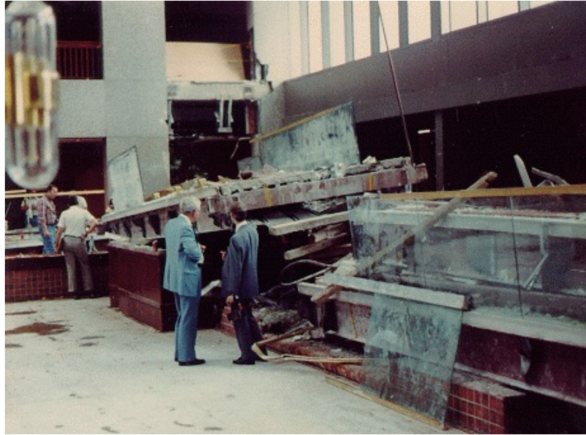
Figure 2: View of the collapsed concrete walkway at the Hyatt Regency that collapsed on the busy walkway below. Credit: Dr. Lee Lowery, Jr., P.E.
