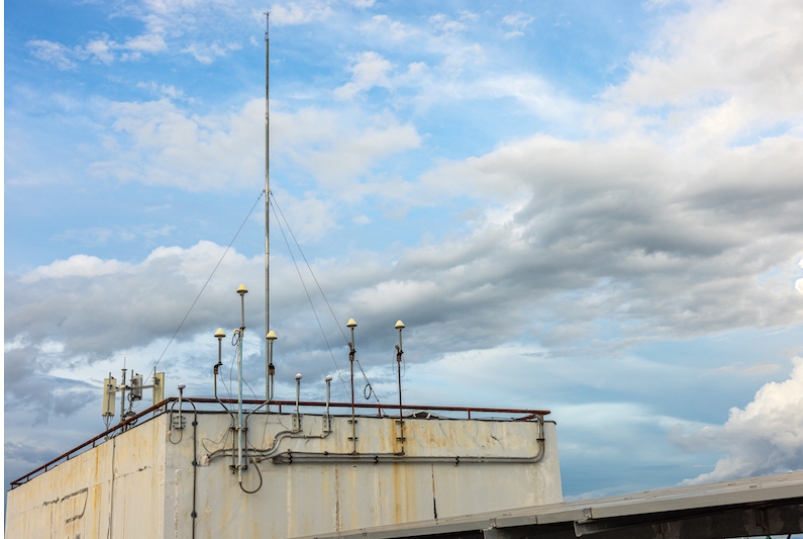
Figure 6: Lightning rod fitted on roof of tall building.
