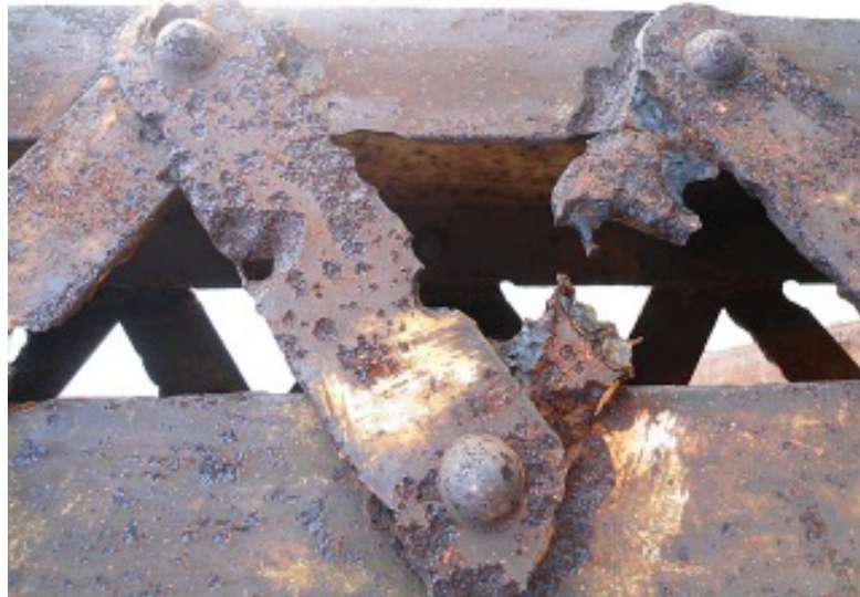
Figure 7: Severe pitting corrosion caused by chloride ions
