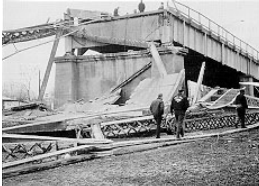
Figure 15: Photograph of the Silver Bridge in Point Pleasant, West Virginia, following its collapse in 1967 (DoT)
